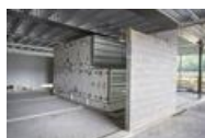
Five Pancras Square (image courtesy of John Sturrock) TROX XCUBE installed at Five Pancras Square (image courtesy of John Sturrock)
