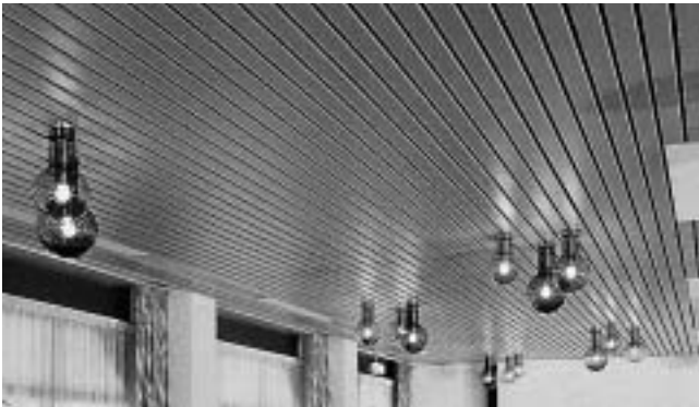
Figure 7: WK-D-P as chilled panel ceiling
