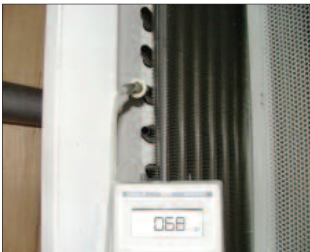
Figure 1: Commissioning a chilled beam by means of measuring the static pressure
